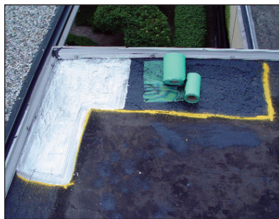
BUILT UP ROOF FLASHING REPAIR Exposed membrane will dry and crack. A simple mastic and membrane repair will prevent leaks and safeguard roof insulation.
