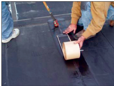
RUBBER ROOF SEAM REPAIR Details and seams are the first to fail. With proactive repairs, the roof life is extended.
