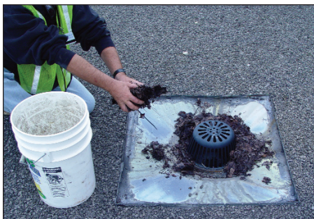
DRAIN CLEANING Annual inspection reports also includes drain, gutter, and general roof cleaning.
