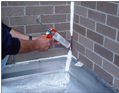
SEALANT REPAIR Typical sealant maintenance is required along walls, counterflashing, and projections.
