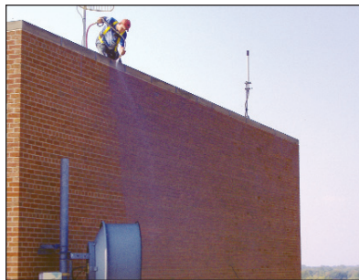
BRICK WALL RESTORATION Powerwashing coping cap and bricks prior to the application of the waterproofing sealant.
