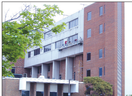
COMPLETE WALL RESTORATION Asbestos wall panels being encapsulated, and window frames removed and replaced, prior to the application of waterproofing materials.
